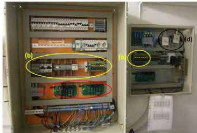
Figure 3. The laboratory installation of the microgrid: (a) The ten CTs, (b) the relays, (c) the ac voltage sensors, (d) the DAQ cards.
