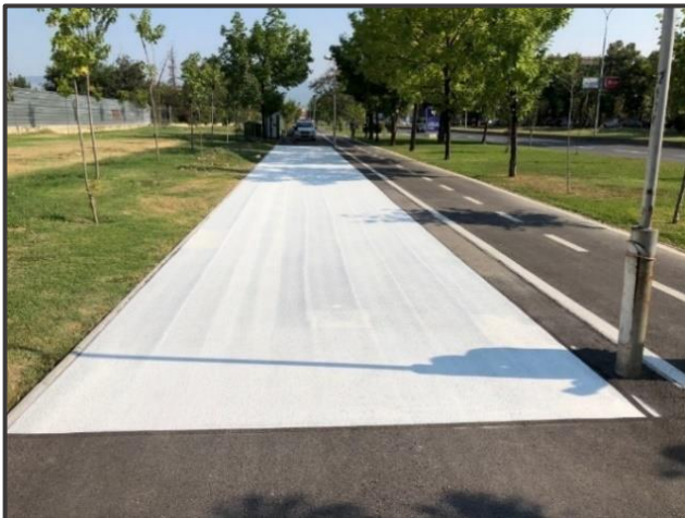
Picture 4: Photo from implementation of the pilot-test of two parts in total area of 225m 2
