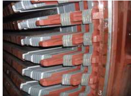
Figure 3. Modernized end part of the magnetic stator core of turbo-generator n.1 in TPP Bitola
