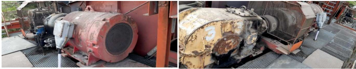
Figure 12: Damaged electric motor and reducer of the coal collection station marked as Js-3
