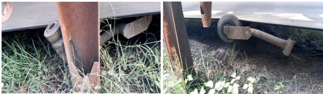
Figure 6: Parts of the load-bearing steel construction in an improper condition due to cracks and fractures from mechanical impacts, installed in the surface mine Oslomej West – Municipality of Kichevo
