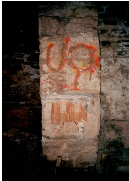
Figure 6: Damaged fresco painting, Church St. Athanasius in Leshok-Tetovo (Directorate for Protection of Cultural Heritage, 2001)
